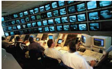
Figure 1: Typical CCTV control room.
